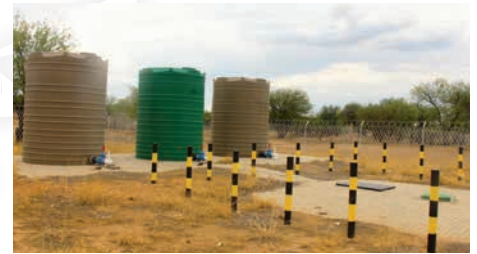
Wastewater plant Tanks
