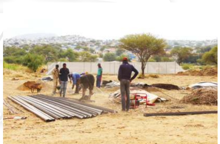
The Farm workers hard at work putting up some infrastructure at the farm
