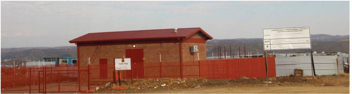
Havana distribution sub-station, one of the three (3) substations that have been erected from which electricity will be distributed to the informal settlements.
