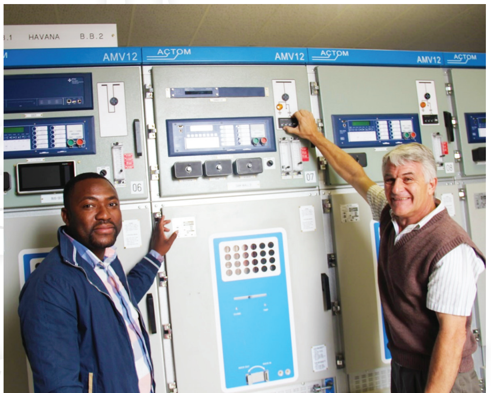
Committed to deliver services to our people...L-R: Mr Leonard Shifotoka Engineer: High Voltage and Medium Voltage Projects Supervision at City of Windhoek and Mr. Struan Steel of ATOM Namibia, the supplier of the 11kV Switchgears for both Havana and Babylon distribution stations
