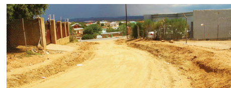
Orinoco Street in Wanahedda, one of the streets that are being upgraded from gravel to tar.
