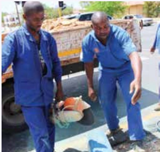
Bulk Water officials hard at work to restore water supply along Sam Nujoma drive.
